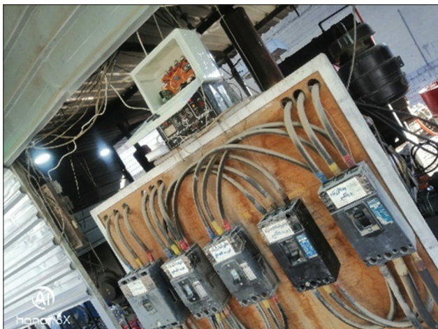
Figure 20: Designed systems at generator
