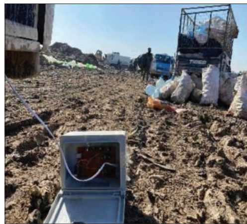
Figure 23: APM at sanitary landfill in Kokjeli area
