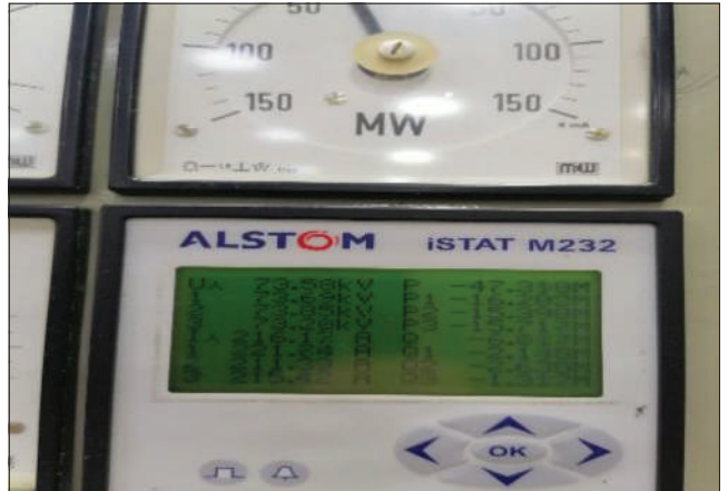
Figure 9: Gauge of current at the station
