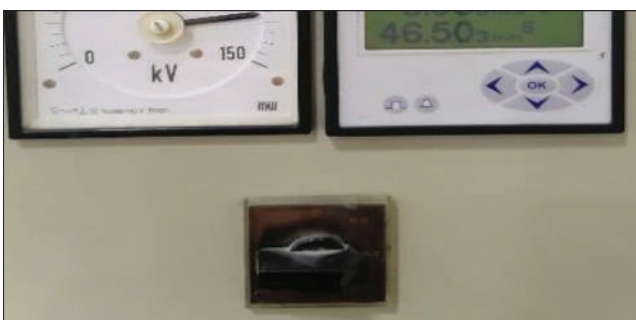
Figure 13: Reading of power at the station
