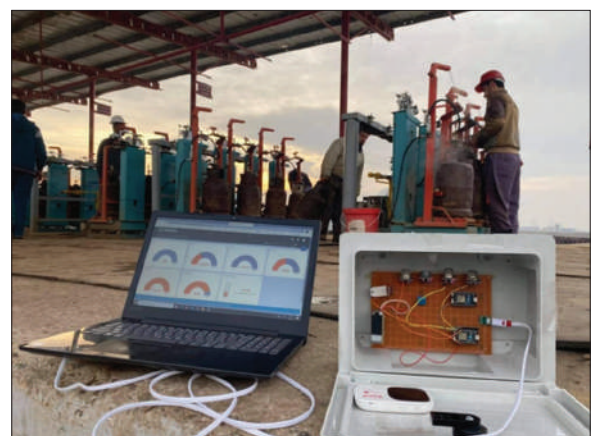
Figure 29: Systems at a gas plant
